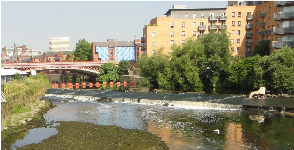
Photo 7: Leeds Dam – debris and damage to boards
