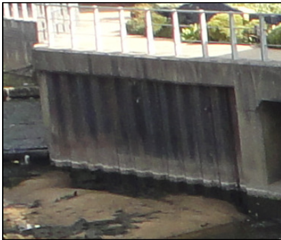
Photo 2: Fearn's Island River Wall, adjacent to weir Photo 3: Turlow Court River wall, adjacent to weir Photo 4: Fearn's Wharf River Wall
