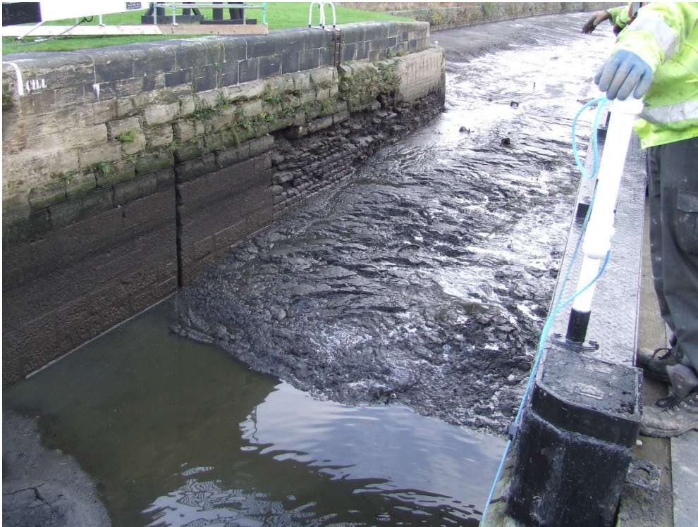
Photo 8: Masonry condition at Knostrop Quay
